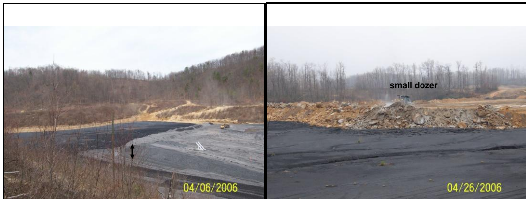
Figure 4: Impoundment cap construction with coarse coal refuse (left) and strip material (right) (modified from Shinavski, 2006).
