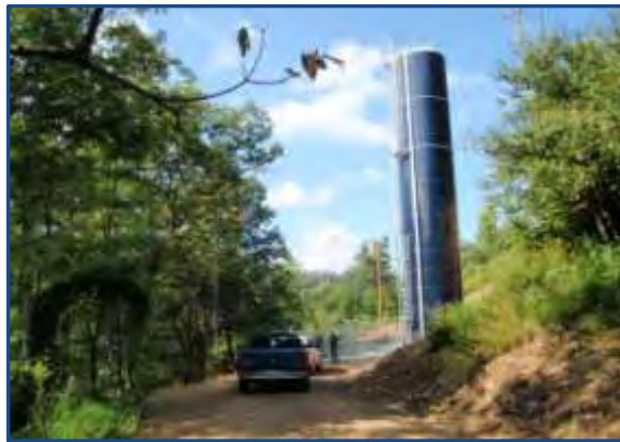
Water storage tank installed under the City of Elkhorn Multi-Site Water Project, Pike County
