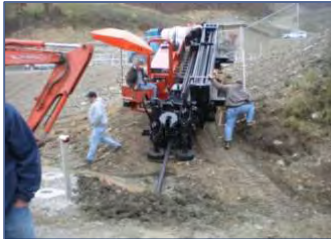
A directional drill used cross a narrow section of Carr Fork Lake in Knott County connecting the Carr Fork KY Highway 1410 Waterline Supply Project and Vicco Waterline Expansion Projects
