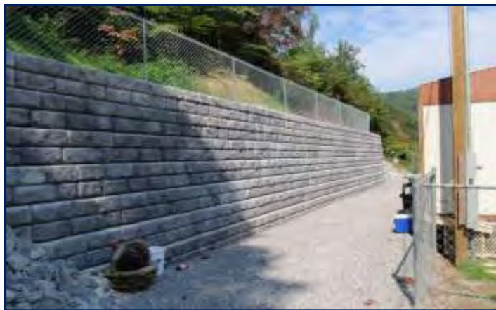
AMLR protecting a home from an unstable hillside resulting from the drainage impacts of an old underground coal mine road at Wheelwright in Floyd County, Kentucky
