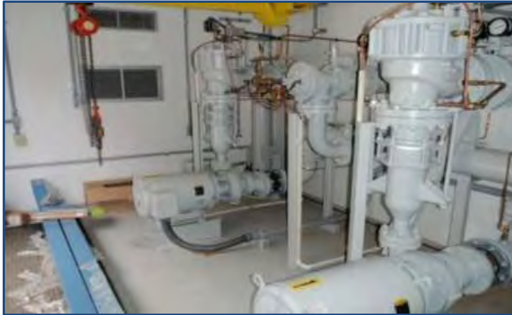
Water line pump station installed under the Irishman Creek Water Supply Project, Knott County
